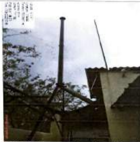
Stack of Boiler approx 11 meter from GL.
