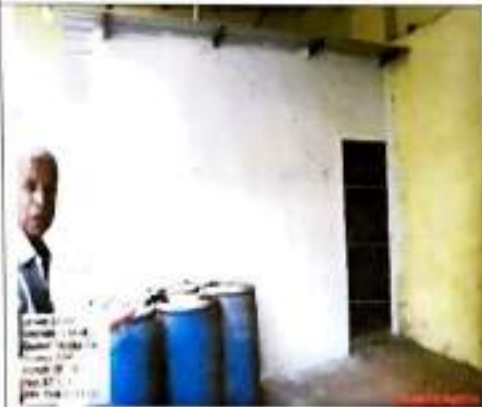
DG Set Room
