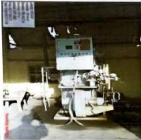
Oil Fired Boiler
